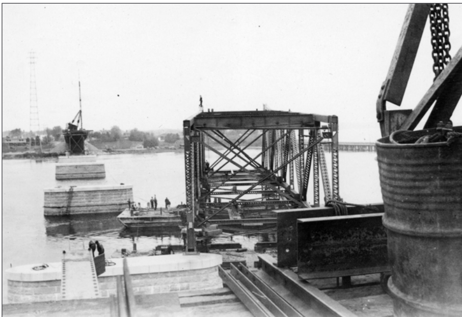
Looking toward the Dover shore as two barges float in a new section.
