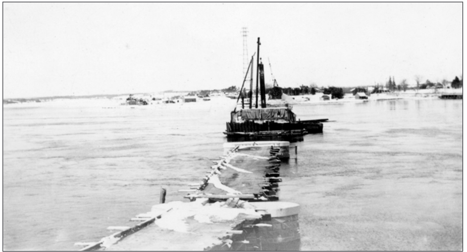
Looking towards Dover with the houses along the Dover shore and Hilton Park. Building bridges over the fast moving tides of the Piscataqua River and Little Bay is not for the faint of heart. Look how close the staging is to the top of the piers and the water level.
